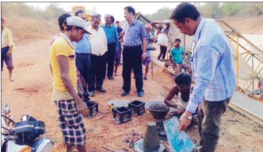
Slump & Cube Testing of CC lining of canal at Subarnarekha Irrigation Project
